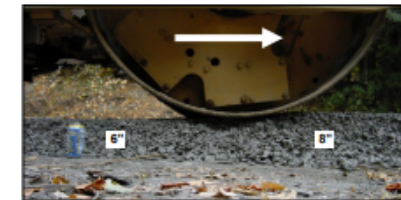
Figure 3 - A roller moving from left to right compacts the 8" lift of loose DSA down to 6"
