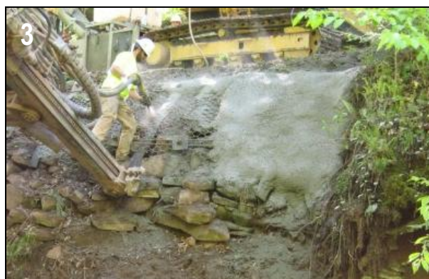
Francis Road: Wire mesh is tied into the exposed ends of the soil nails, then a “shotcrete” facing is added.
