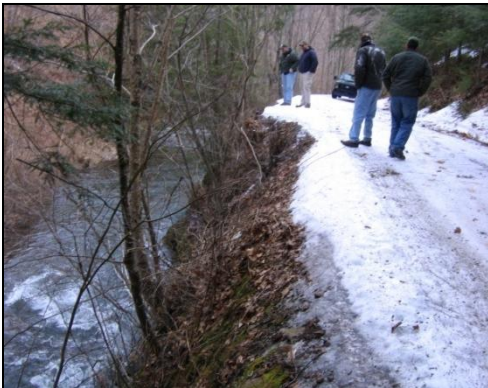
Francis Road (before): The bank instability here was caused by the proximity to the stream.
