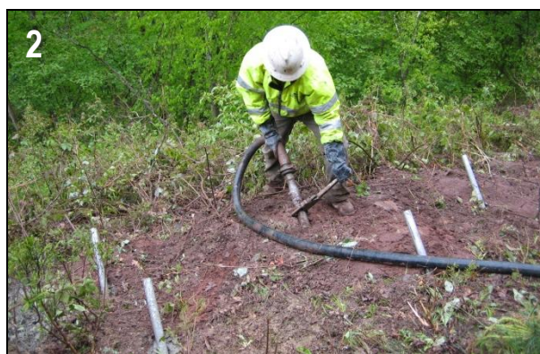
Slate Run Rd: Grout is pumped through a hollow soil nail to fill the hole from the bottom up.
