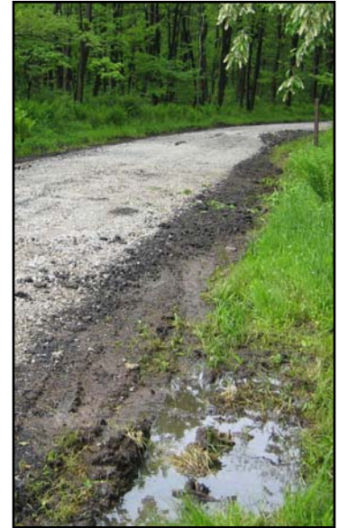
Much of the existing road was saturated for extended periods of time due to an impermeable clay layer.
