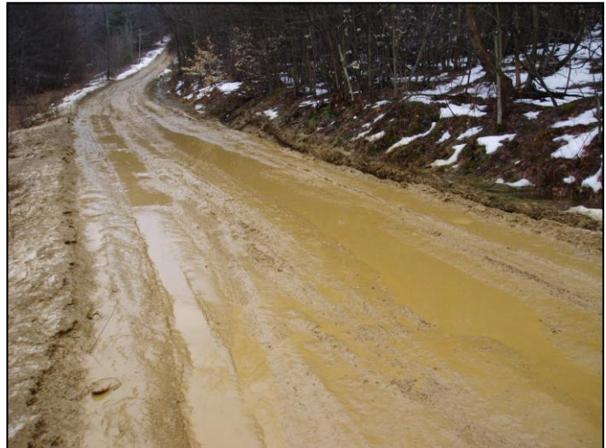
Figure 6.2: This image, taken in the Grunder watershed in late March after a natural rain event, illustrates the effect of poor road material, excessive moisture, and vehicle traffic on sediment generation. (photo courtesy ANF)
