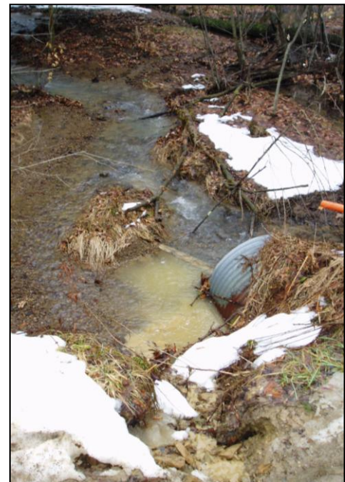
Figure 1.1: Example of the effect of road runoff on aquatic ecosystems. This image, taken in the Allegheny National Forest adjacent to site "C" in this study, shows road runoff entering Grunder Run at a crossing. (photo courtesy ANF)
