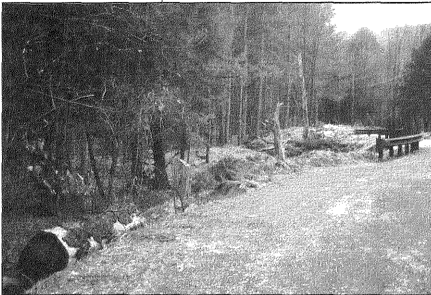
AFTER: Earth mounds were created and covered with native vegetation to retain stormwater so that it could be slowly released into nearby woodlands.
