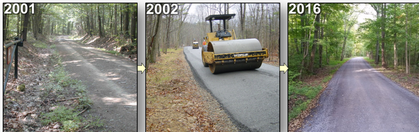
This 15 year old project in Huntingdon County illustrates the long-term road improvement practices implemented by the Program, in this case filling the road profile, adding shallow crosspipes, and Driving Surface Aggregate.
