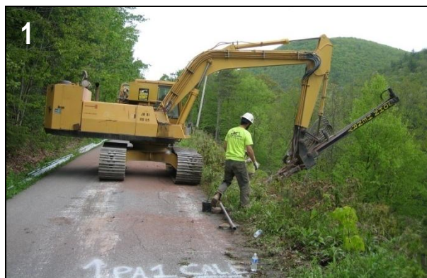
Slate Run Rd: Soil nail holes are drilled into the road slope.
