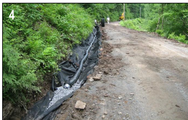
Slate Run Rd: 2,000 feet of underdrain was installed due to the many springs and seeps that kept the road area saturated for much of the year.
