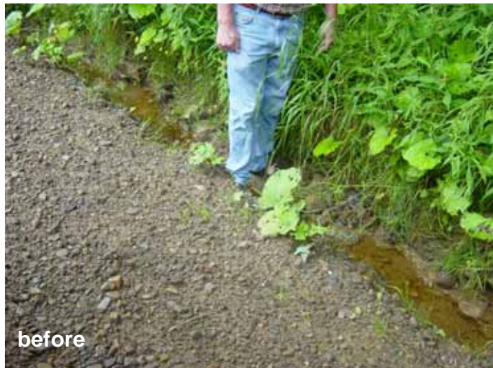
before Before: Limited drainage outlets meant road drainage concentrated in narrow deep road ditches that eroded deeper and deeper over time.
