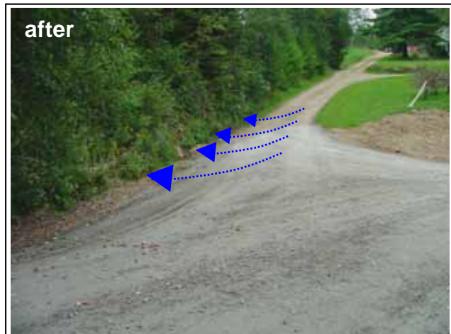
After: This driveway was re-shaped with fill material to direct water coming down the driveway into a pipe and keep it from spilling onto the road itself.
