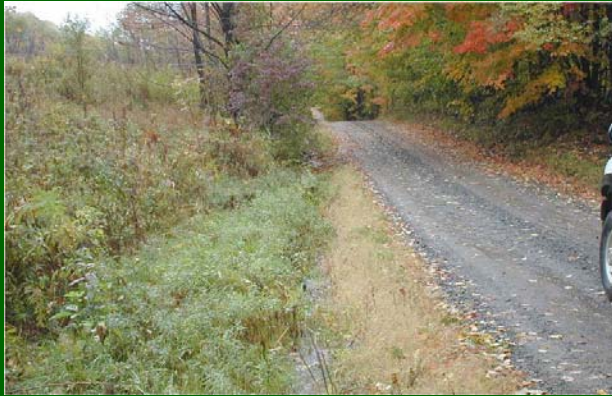
Figure 3. BEFORE filling: Note ditch on the left and high bank to the right of road.
