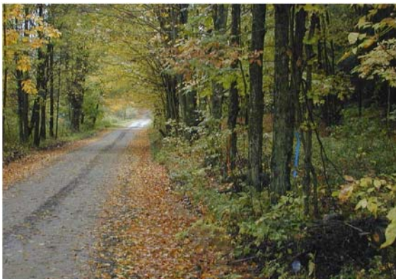
Figure 1. BEFORE: Depressed road without crosspipes, road collects and carries water.
