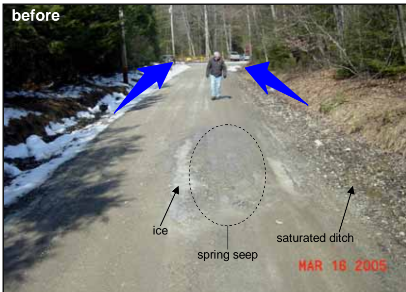
Photo 1. Notice the ice in the middle of the road from a spring seep. The entrenched road profile made it impossible to get water or snow off of the road.
