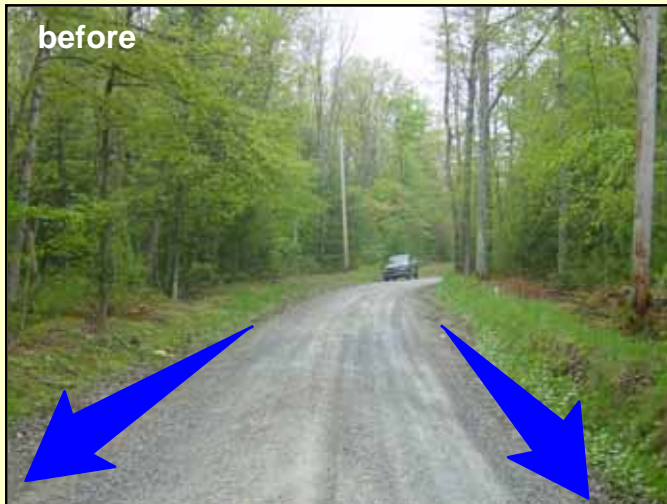
Photo 3. The entrenched road traps water in the road area and conveys it down to the stream. Note the elevation of the road relative to the utility pole on the right compared to Photo 4 .
