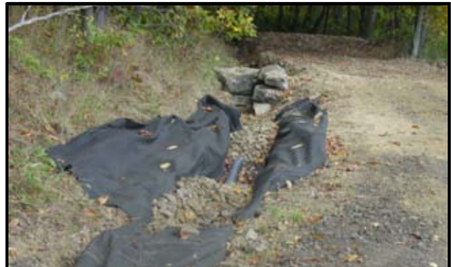
Photo 3: Underdrain installation in progress. Underdrain continues under road and outlets separately from crosspipe.
