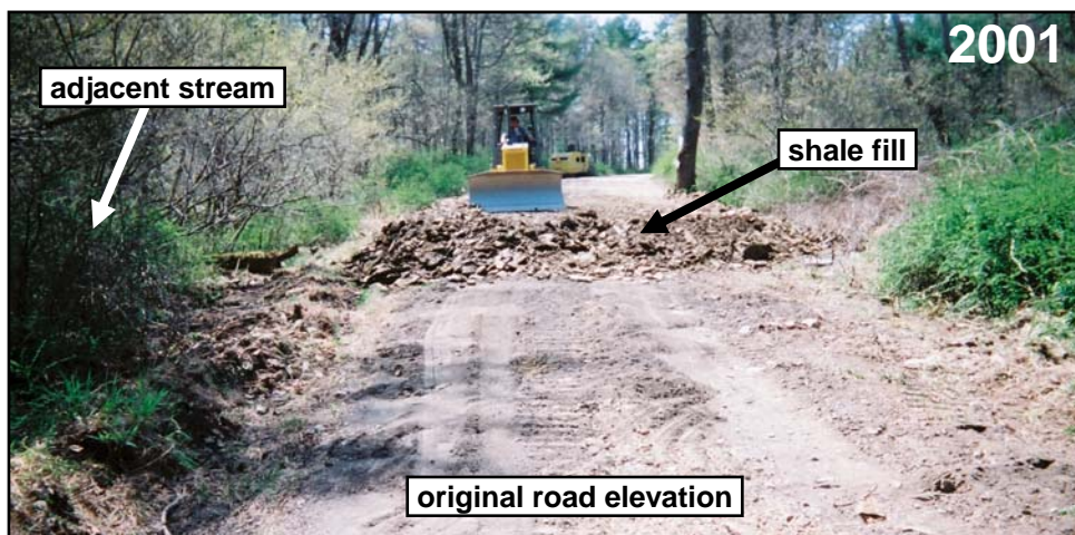
Photo 1. Spruce road was filled with up to 2' of shale in places to provide a better road base and elevate the road above the adjacent stream.
