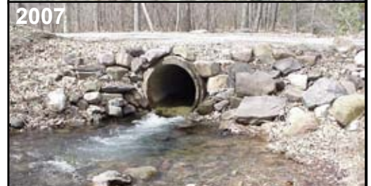
Photo 3&4. Before and after of concrete pipe. Note how pipe is scoured before, protected after.
