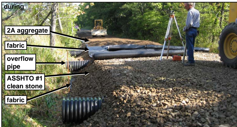
Photo 3. French mattress with overflow pipe installation in progress. 600' of DSA will be placed over the site after the mattress is given some time to settle.
