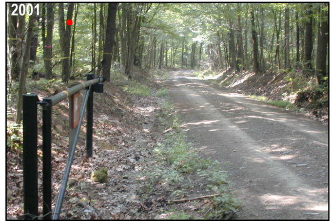
BEFORE. Existing entrenched roadway traps drainage and transports it to stream around bend.
