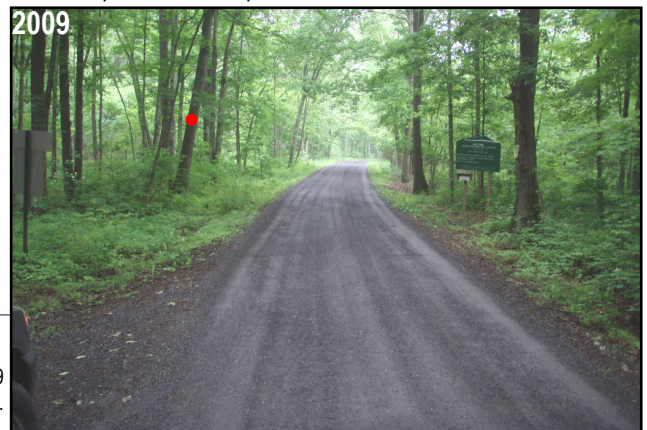
AFTER. Raising the road provided a long-term solution to the runoff issues on Red Rose Road.
