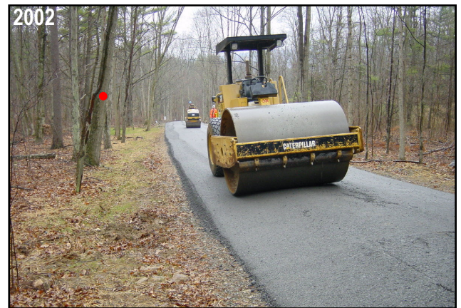
DURING. Driving Surface Aggregate is placed 8" deep using a motor-paver and compacted to 6" with a roller.
