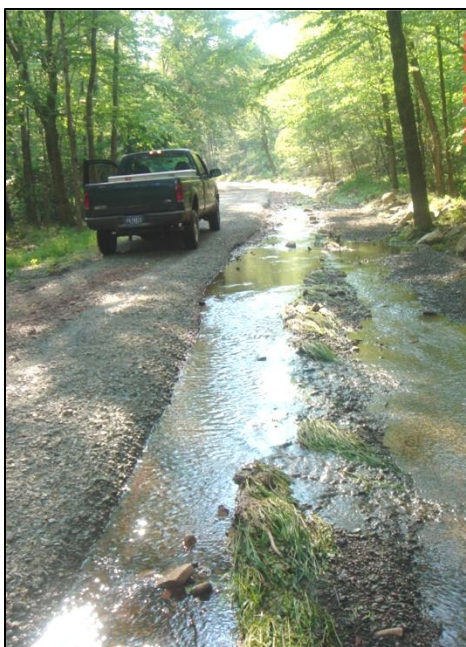
Tannery Road (before): Shown after a flow event that overtopped the stream pipe and ran down the road in 2006.
