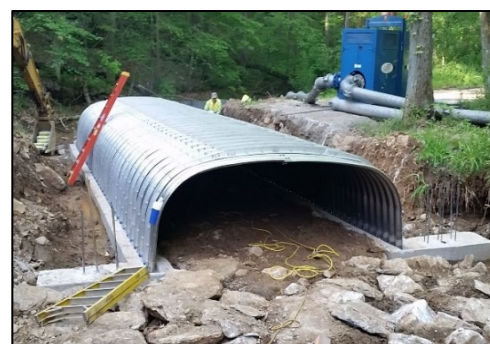
Bottomless arch pipe (York)
