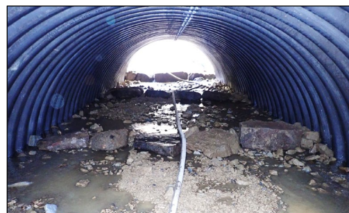
Photo 3: Grade control placed inside of a 15' wide arch pipe before placing final streambed.
