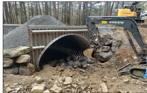
Photo 1: Placing grade control material in a 15'w x 10'h pipe arch (squash pipe).
