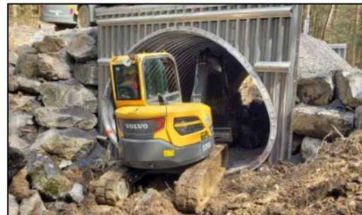
Photo 1: Placing larger material in a 15'w x 10'h pipe arch (squash pipe).
