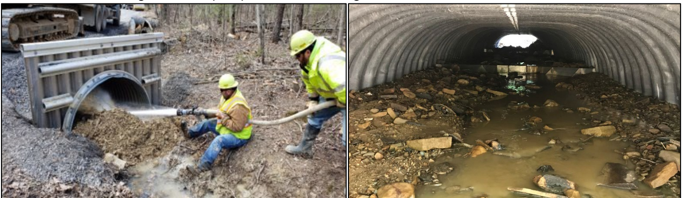
Figure 6: The photo on the left shows washing of fine material into a 6'w x 4'h pipe arch (squash pipe) using a fire truck. The photo on the right shows the washing process between tanker loads and view of a baffle grade control.
