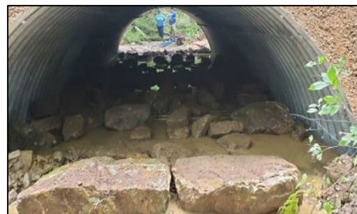
Photo 4: Large material placed in a 12'w x 6'h arch pipe before placing streambed.
