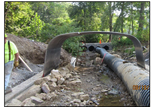
Assembly of a 15' w x 6' h bottomless arch pipe on cast-in-place footings (Juniata).
