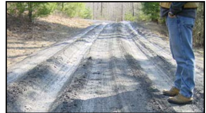
Rutting due to clay content (high plasticity index) in a surface aggregate
