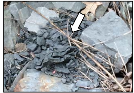
Disintegration of “unsound” rip-rap due to one year of freeze/thaw cycles.
