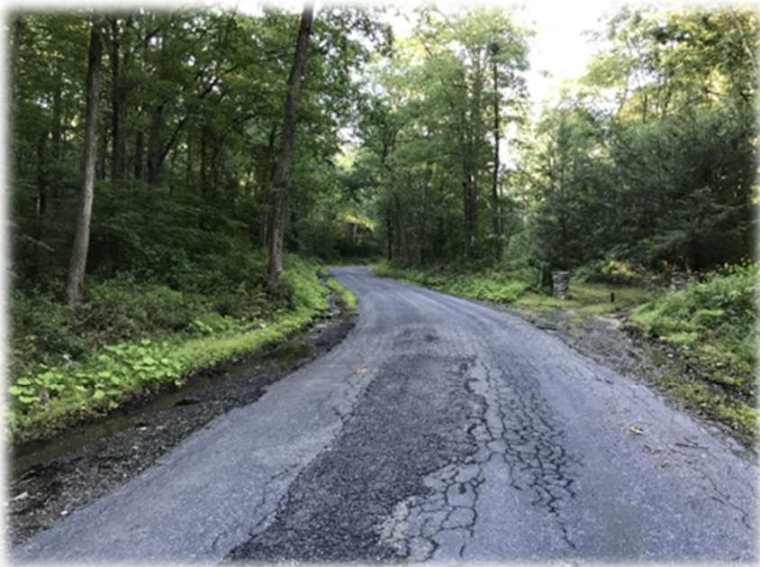
Before picture of cover photo project. 800 feet of underdrain and a 500 foot French Mattress served to dry out this saturated roadbed. Paving was done in-kind.
