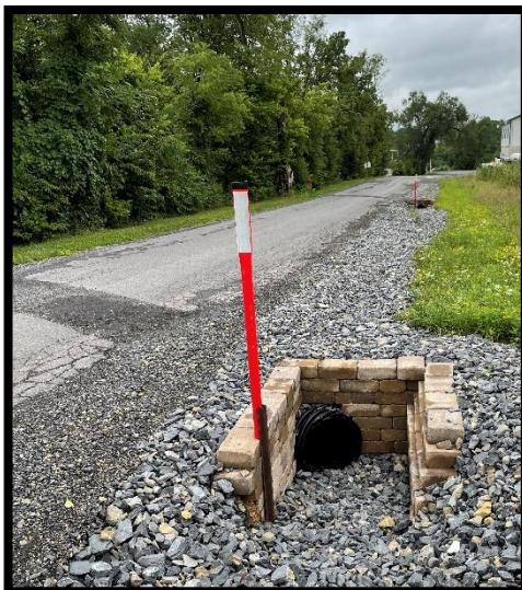
Cross pipes are commonly used in DGLVR projects to direct water away from the road and nearby streams.
