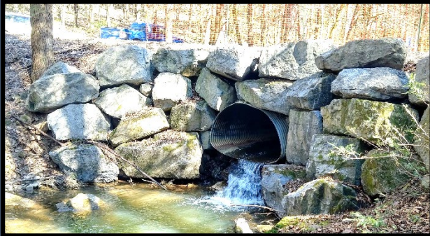
Erosion and aquatic barrier at undersized pipe outlet
