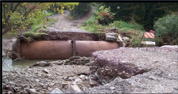
A clogged pipe inlet led to a complete road washout.
